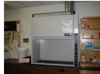
Fume hood with Galvanized ductwork.
