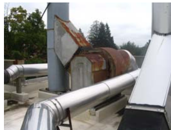
Abandoned Exhaust fans.
