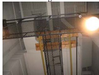
Ceiling hung AHU. Ladder up to service platform.
