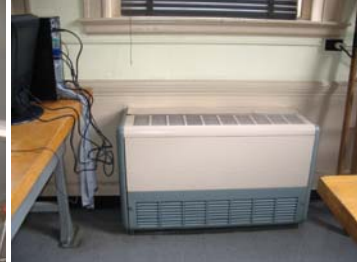
Original Unit Ventilator.
