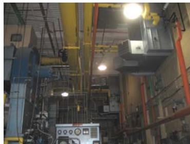
Boiler Room Unit heater
