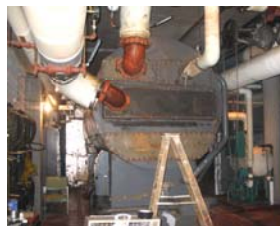
600-ton steam absorption Chiller. Low Eff.
