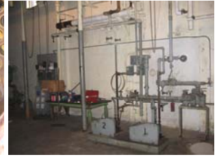
#2 Fuel oil transfer system.
