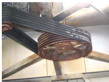
Corroded Fan sheave.
