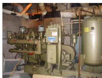
Industrial capacity air compressor set.
