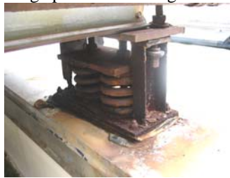
Corroded spring supports.
