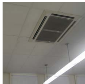
Ceiling Ductless AC.
