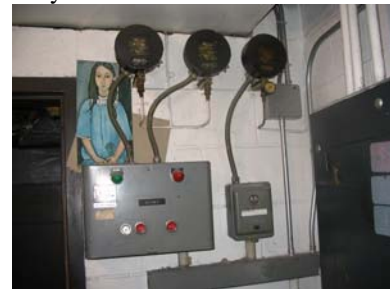
Very old, original controllers.
