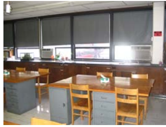
Window AC units, no make-up air.
