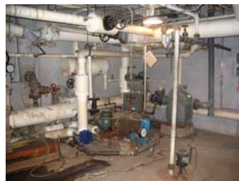
Mechanical room with steam PRV, Gas meter, converter, and ejectors.
