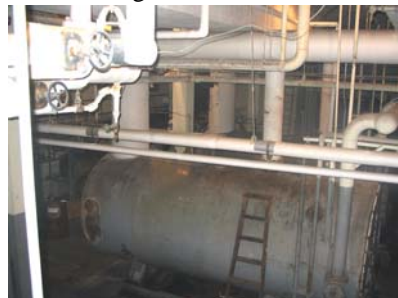
(2) 250 HP Ray FT Boilers.
