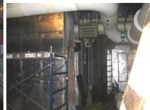
Built up AHUs in good shape.
