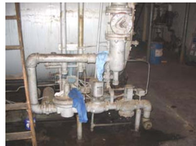
Dual fuel capability but gas was never connected.
