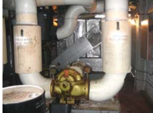
Pumps in fair shape.
