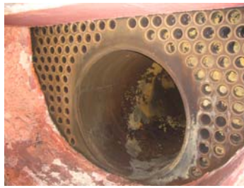
Boilers are in very poor shape.
