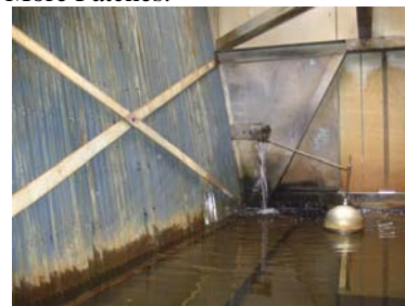
Cooling tower cold sump.
