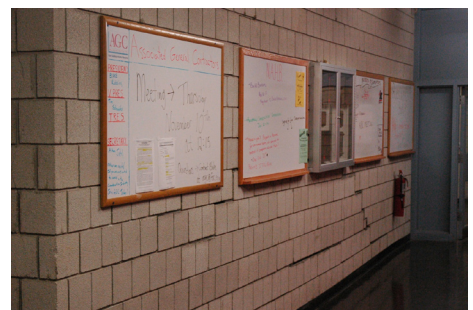
Structural Problems Plague Many Buildings on Campus, Like the Conlon IA Building Pictured Above
