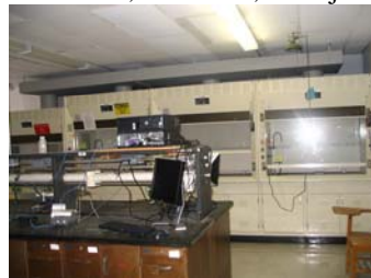
Gang of 3 FH's w/ improper Ductwork.
