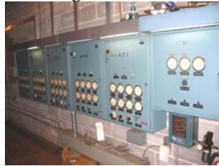
Original pneumatic control panels.
