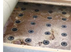
CT Corroded through warm basin
