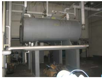
Feed water system.
