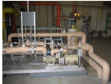
Fuel Oil Transfer Pumps.
