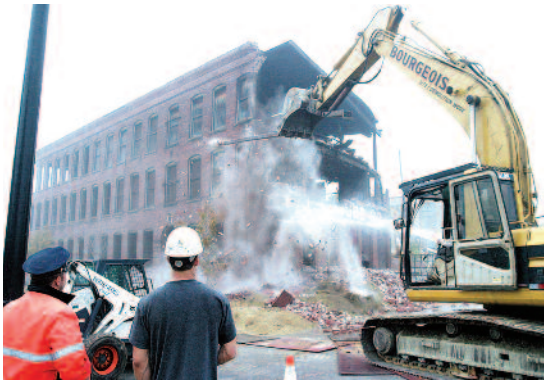
Years ago, the North Street project began with the demolition of several former mill buildings.
