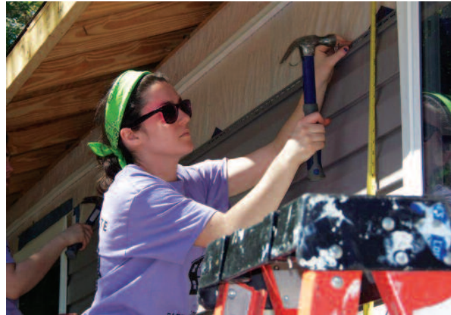
More than 20 students, including Samantha Kaplan, above, traveled to Florida for the campus' annual alternative spring break trip to volunteer for Habitat for Humanity. Work crews helped repair and build homes during their week down south, and also had time to soak up a little sunshine.
