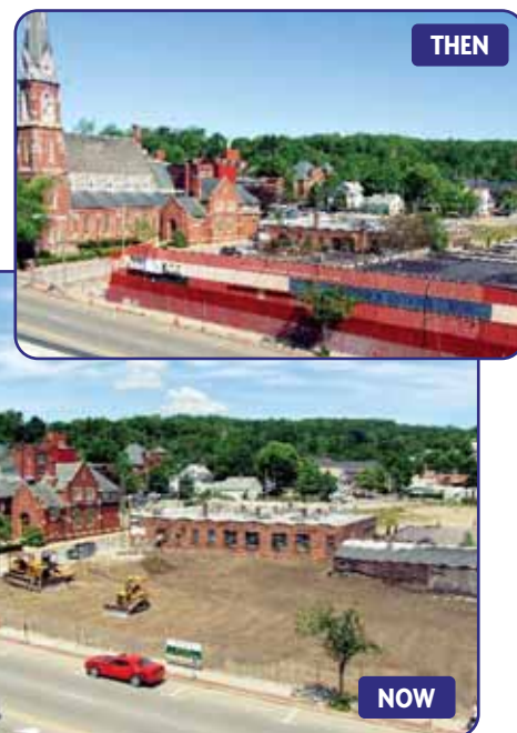
The building at Main and North streets as it appeared at the start of demolition in early May and then razed.
